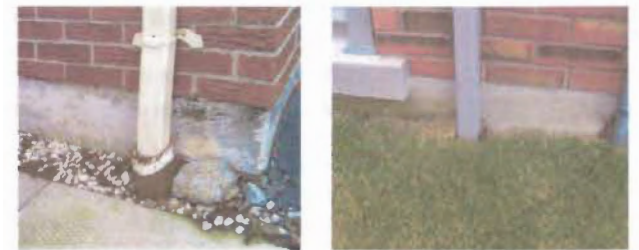
These downspouts are connected to the underground municipal sewer system
