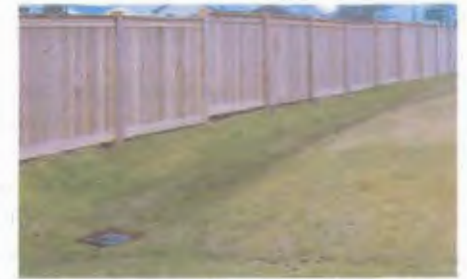
Rear-yard swales direct flows to a catch basin in this image. Rear-yard catch basins and swales shouldn't be covered or filled in with backyard sheds, fences or other structures, and rear-yard catch basins should be kept clear to reduce backyard flooding.
