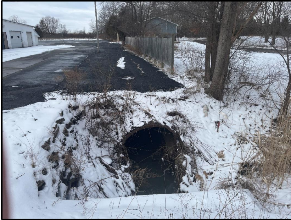
Photograph 4. Piped Drain Under Parking Lot Upstream of the Box Culvert Crossing at Niagara Street March 2023, Looking Upstream
