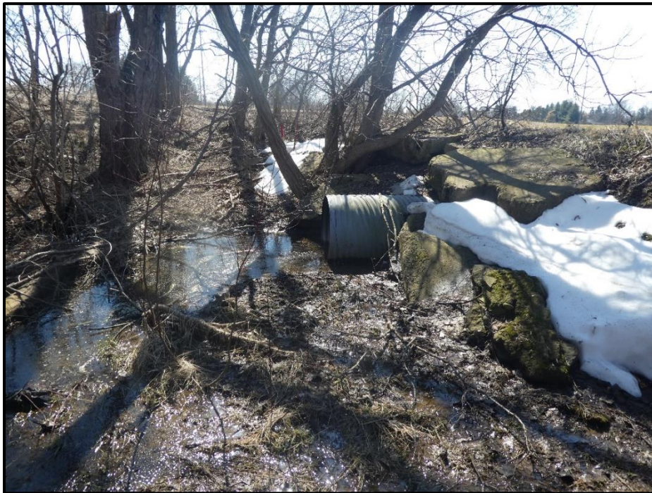
Photograph 3. Area 1 Soccer Field Piped Section Outfall to Channel of the Drain March 2022
