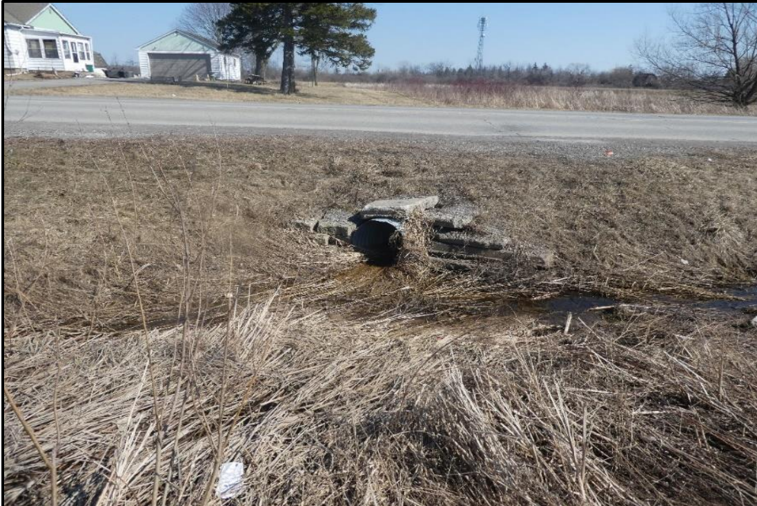
Photograph 11. Drain at Rice Road Culvert Crossing; Looking South Downstream to Rice Road in March
