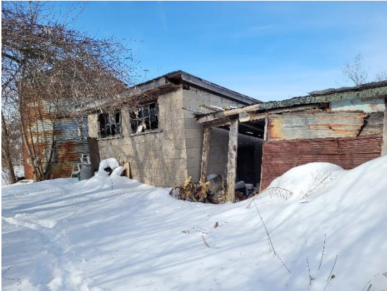
Picture 19: View of the sheds to the north of Site Building A, facing northwest.
