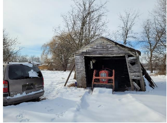
Picture 20: View of the shed to the west of Site Building A, facing west.
