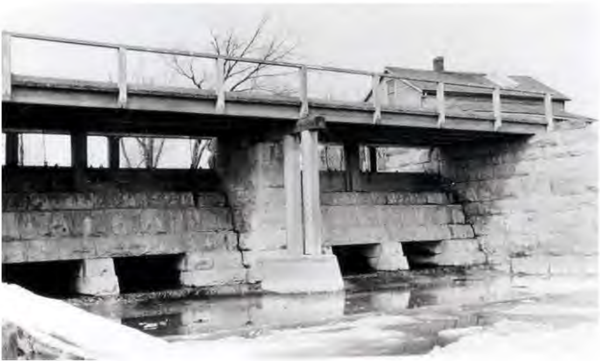
Figure 13 Spillway of the Feeder Canal into the Welland Canal at Welland, ON 1924
